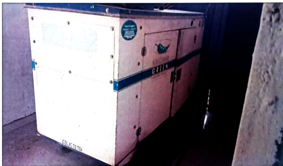
Figure 2.1:- DG set on the college campus
